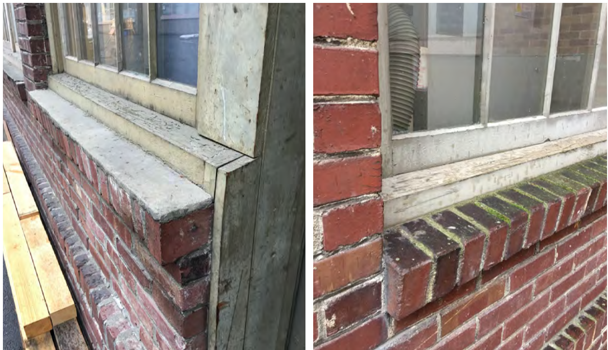
Figure 47. 1909 window sill and sub sill detail with cement wash (above left) and 1920 window sill and sub sill detail (above right).
