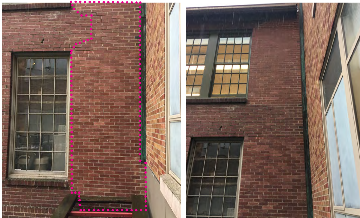
Figure 46. West facade, south end, details of 1958 brick rebuild and window removal as part of the MEB end wall connection.
